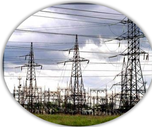
Karadum substation has 110\35\6kV S= 16mVA
