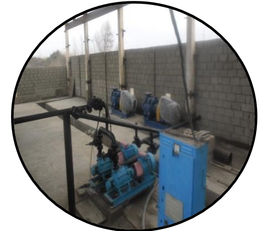
Water supply Pumping station FEZ "Panj"
